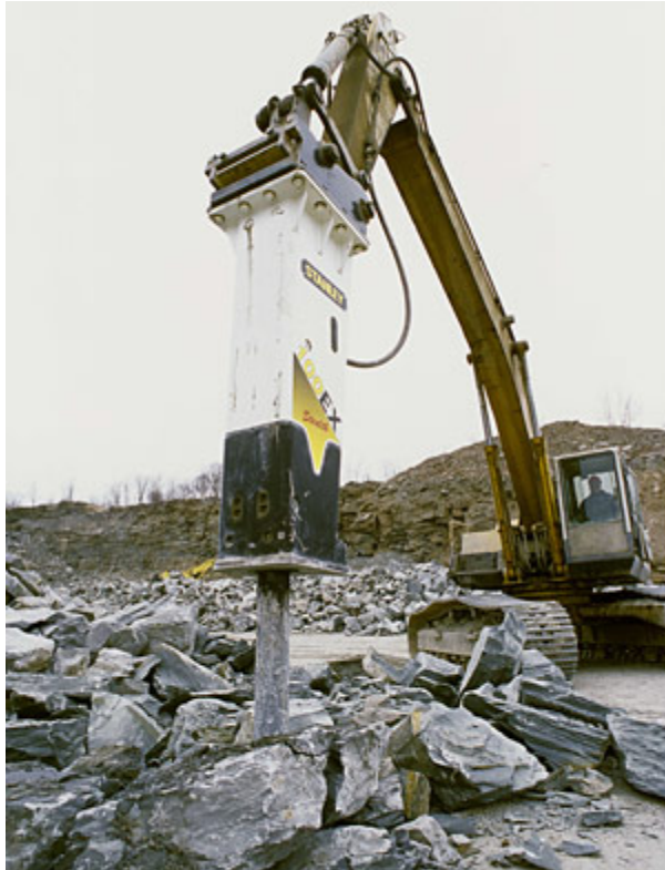
The new breaker reduces material at a rate of 80 to 100 tph.
